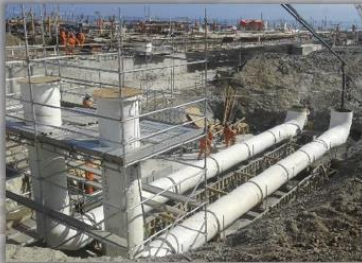
Desalination plant: BHP Coloso project (2016-2017)
